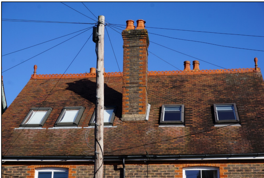
Fig. 10: Two hole hexagonal crest ridge tiling with finials and red brick chimney stack quoin, Hazelwick Road.
