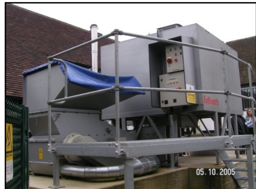
Figure 9: A biomass boiler fuel feed system (ecsc)
