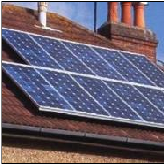
Figure 4: Solar Photovoltaic Panels ( www.solarcentury.co.uk )
