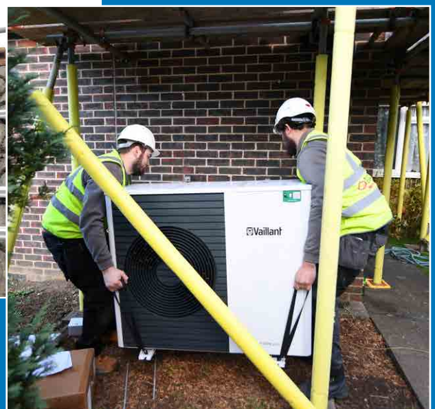
Air source heat pump
